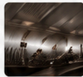
CHIMNEYS & HOOD FILTERS
